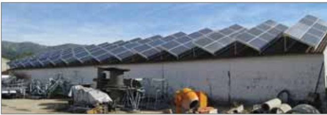
Figure 13- photo of farm installation in Spain
