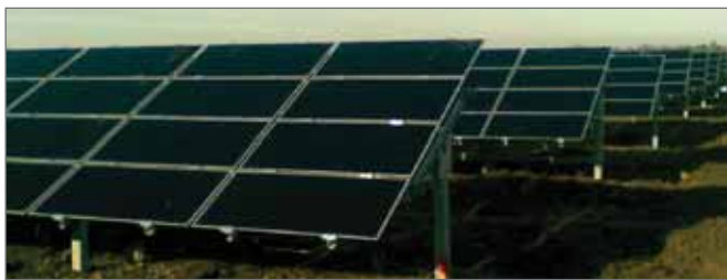
Figure 18 – photo of typical field installation
