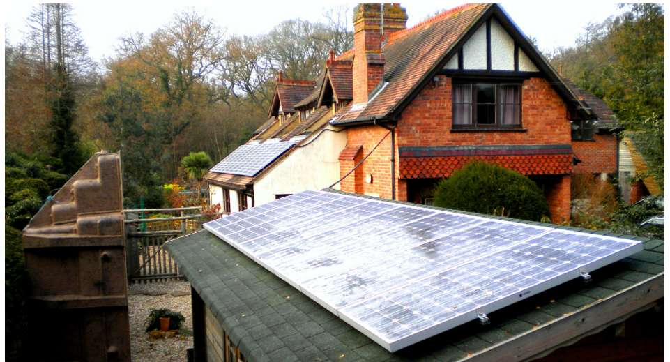
A 3.3 kWp installation consisting of one string with 18 modules that spreads across two roofs with two different slopes: 25° and 40°. The string is connected to a SolarEdge SE3300 inverter.
