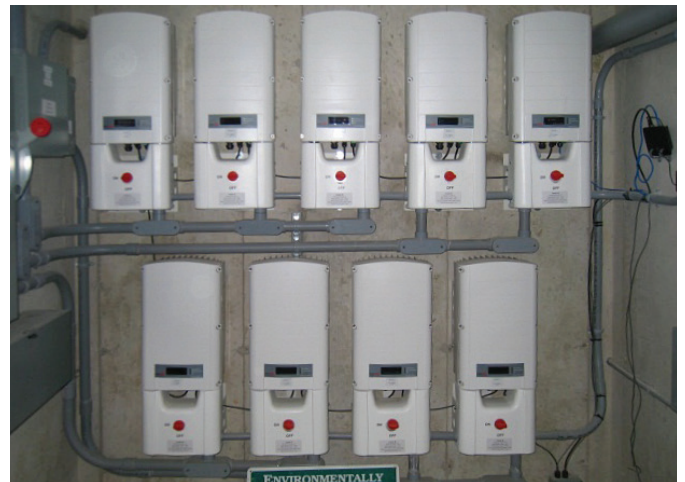
Figure 3: The SolarEdge inverters in the Donkers' utility room. Photo by Sashaan Solar
