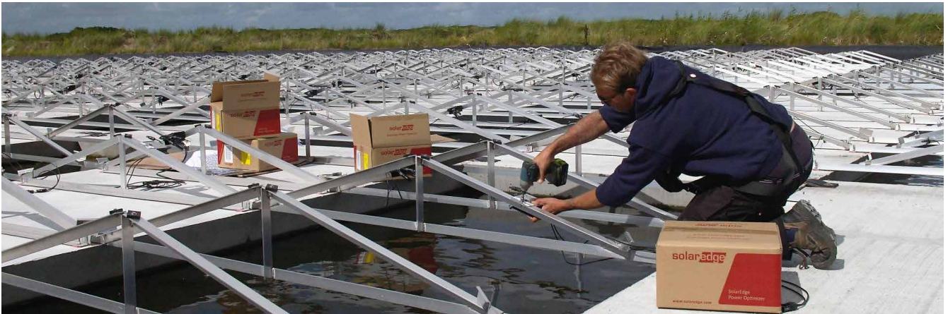
The PV installation was set on a concrete pontoon above the reservoir.
