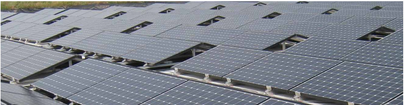
The floating installation covers the majority of the water surface, reducing fresh water evaporation and growth of algae on the water surface.
