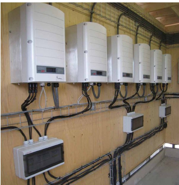
24xSE27.6K inverters are installed next to the pond.
